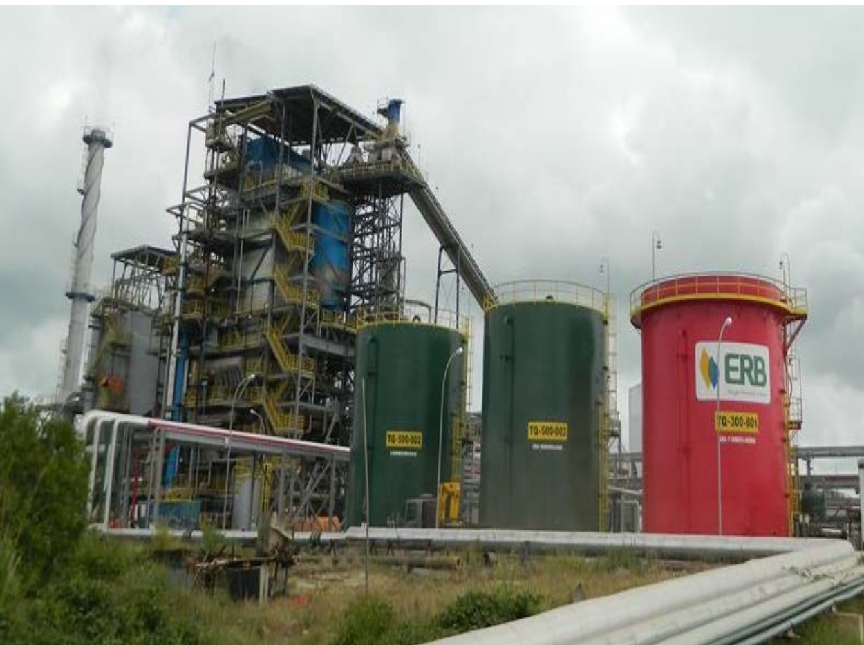
ERB biomass CHP plant in Candeias in Salvador, Bahia, Brazil
